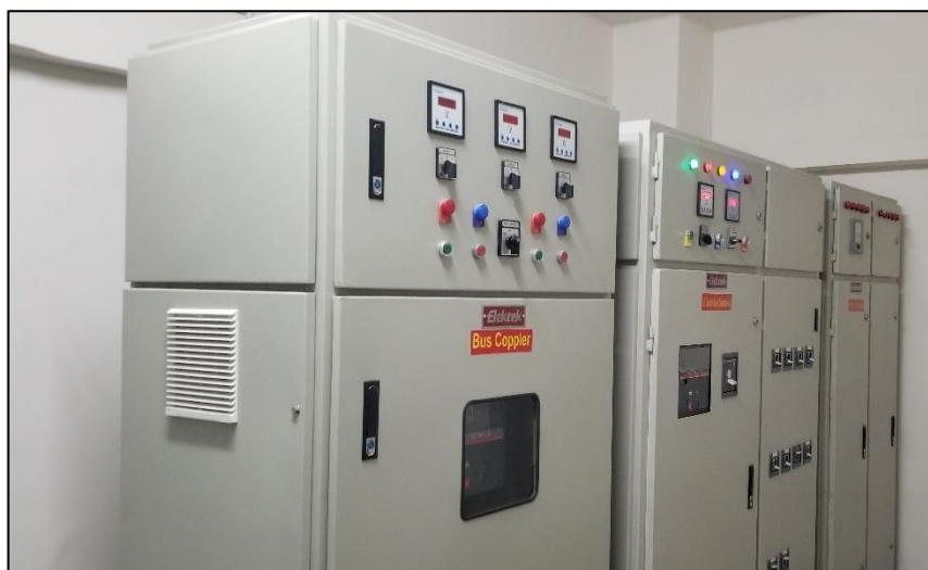
Sub- station installed at the DDM Building
