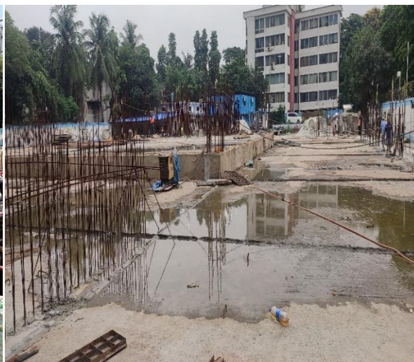
Curing work after floor, ramp, and lift core casting in level B1
