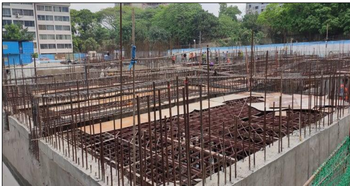
Centering and shuttering work in on-going for the beam and roof of Basement -1 (B1)
