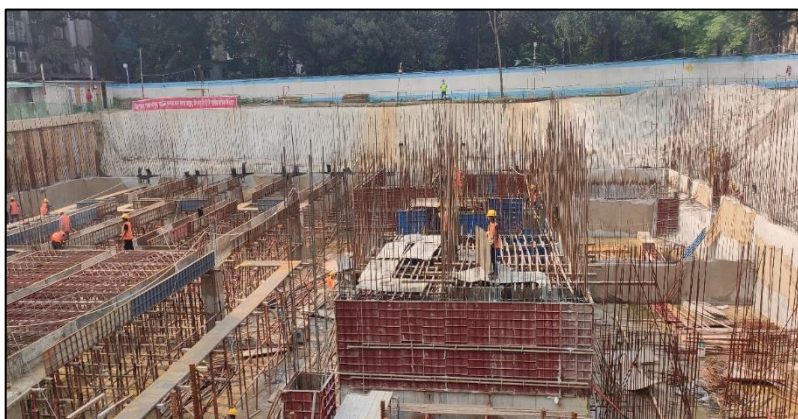
Shuttering and centering work on-going for the beam and roof of Basement -2 (B2)
