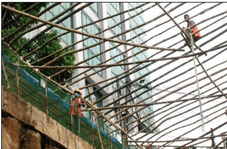
Working at height without helmet, and safety gear
