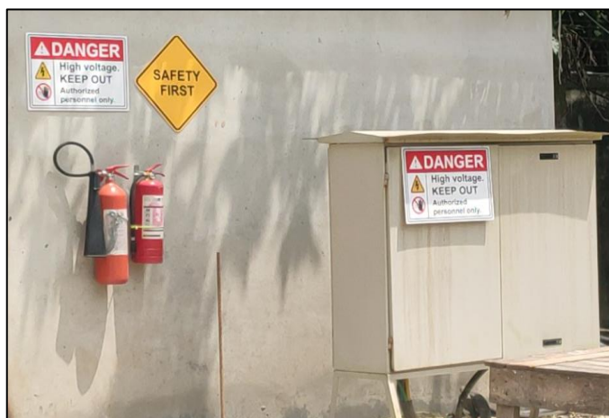
Displayed Safety Instruction and fire extinguisher
