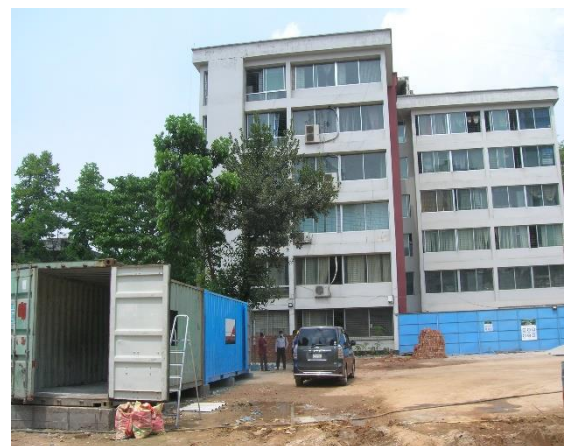
Residential apartment building abutting work site without any sound or dust barriers.
