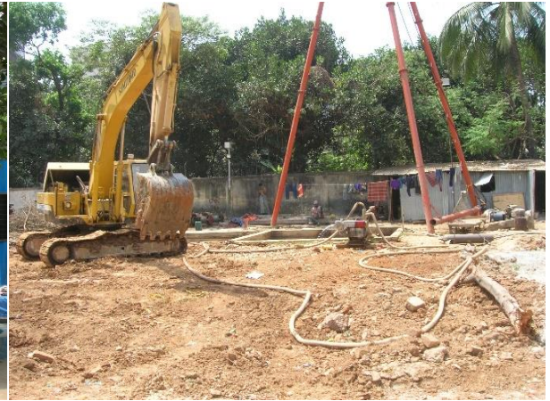
Pile foundation work in progress, but hoses and debris littered about site.
