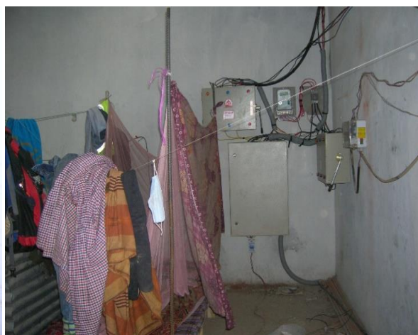
Risky electrical installations at camp-1 jeopardizing workers safety
