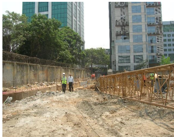
Lack of properly indicated, safe walkways or any signs warning of safety hazards.
