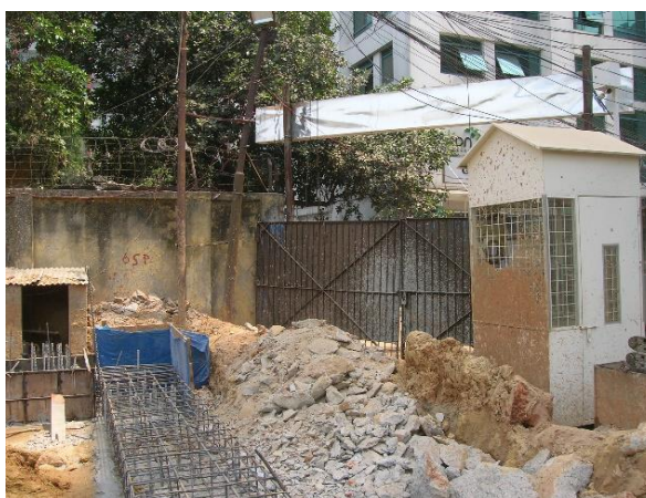
Haphazard placement of concrete and other solid wastes on-site. Lack of proper disposal off-site.
