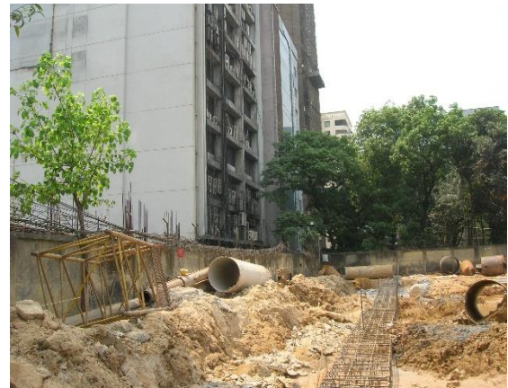
Disorganized and improper placement of large supplies, posing safety hazards.
