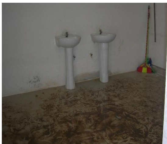
Unhygienic bathroom floor, no hand soap or sanitizer. Lack of showers or clothes-changing area, or temporary toilets
