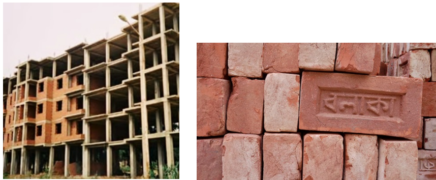
Figure 8-27: Very typical multistory building in Dhaka with unreinforced masonry infill. The building also has a soft story at the bottom.
