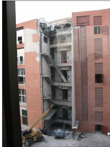
Damage to Chilean buildings and other structures caused by the February 2010 earthquake was commensurate with the severity of the earthquake
