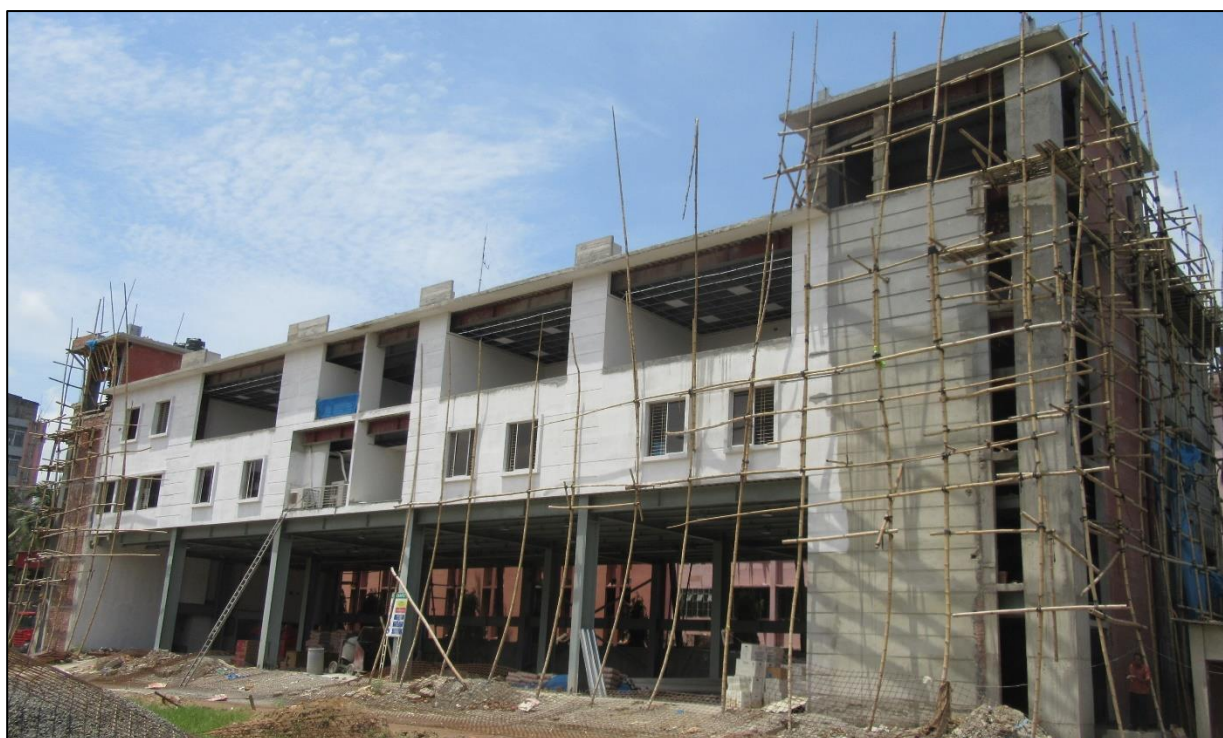
Figure 1: Construction of Warehouse and Command and Control Center of FSCD in Mirpur-10
