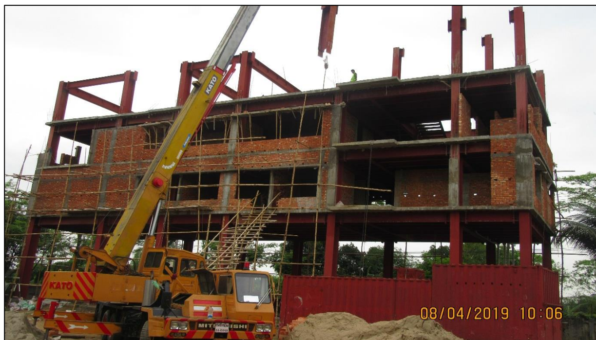
Figure 2: Construction of Command and Control Center and Warehouse of FSCD in South Surma, Sylhet.
