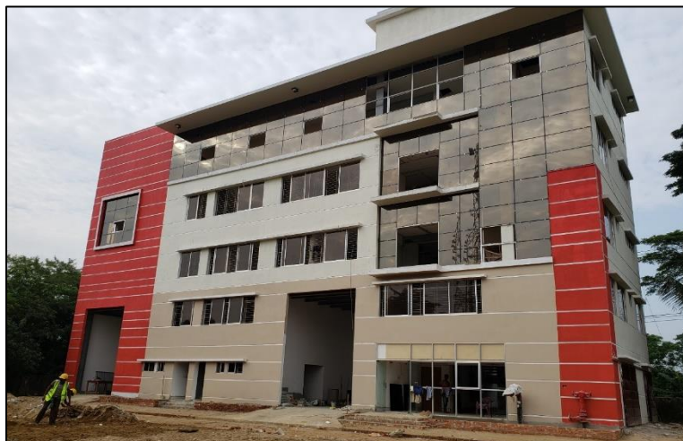
Command and Control Center with Warehouse of FSCD at South Surma, Sylhet.
