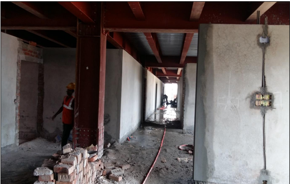
Figure 2 : Construction of Warehouse and Command and Control Center of FSCD in Mirpur-10
