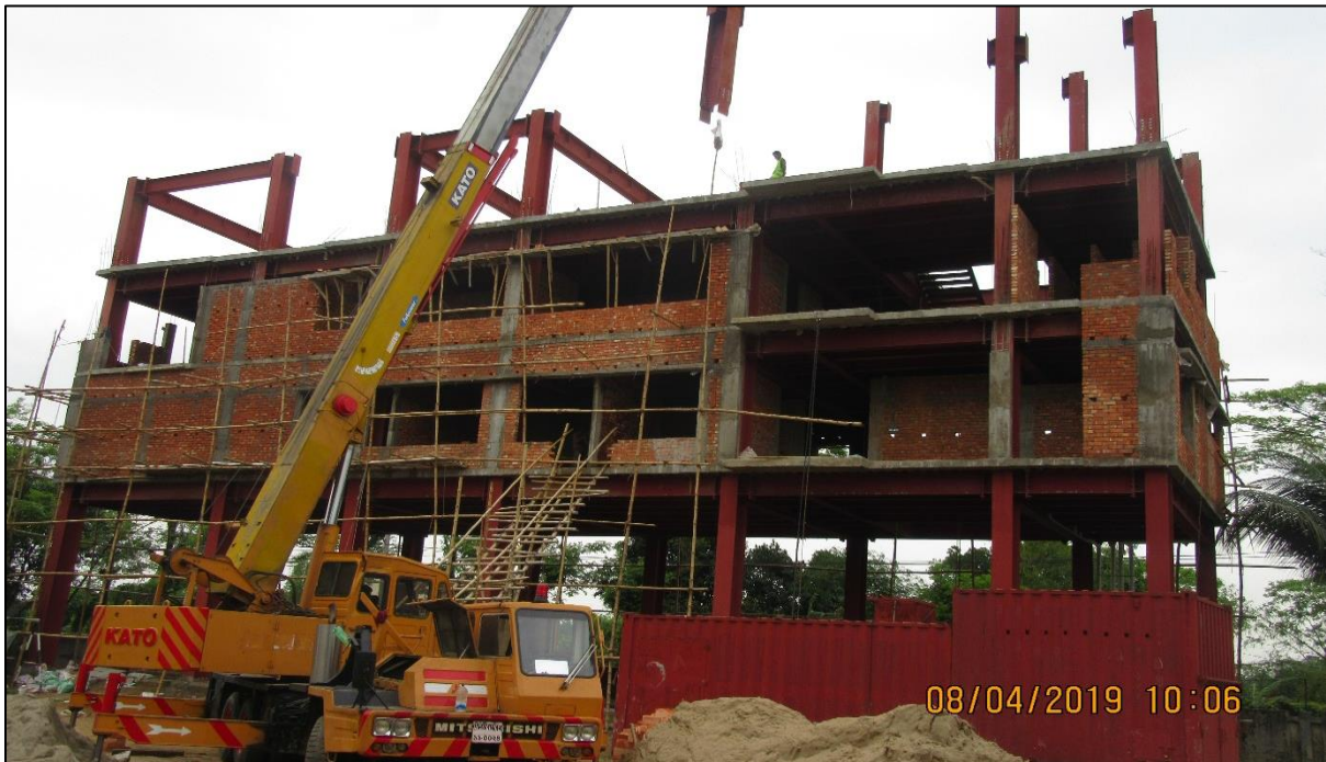
Figure 5: Construction of Command and Control Center and Warehouse of FSCD in South Surma, Sylhet.
