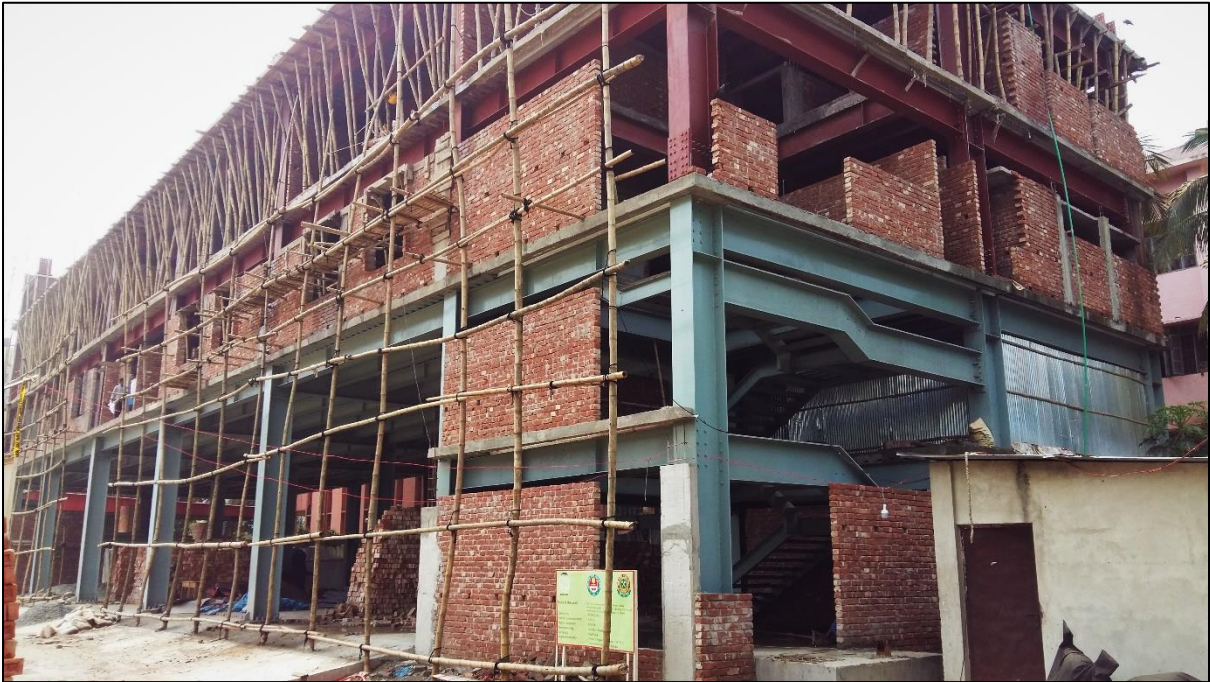
Figure 1: Construction of Warehouse and Command and Control Center of FSCD in Mirpur-10
