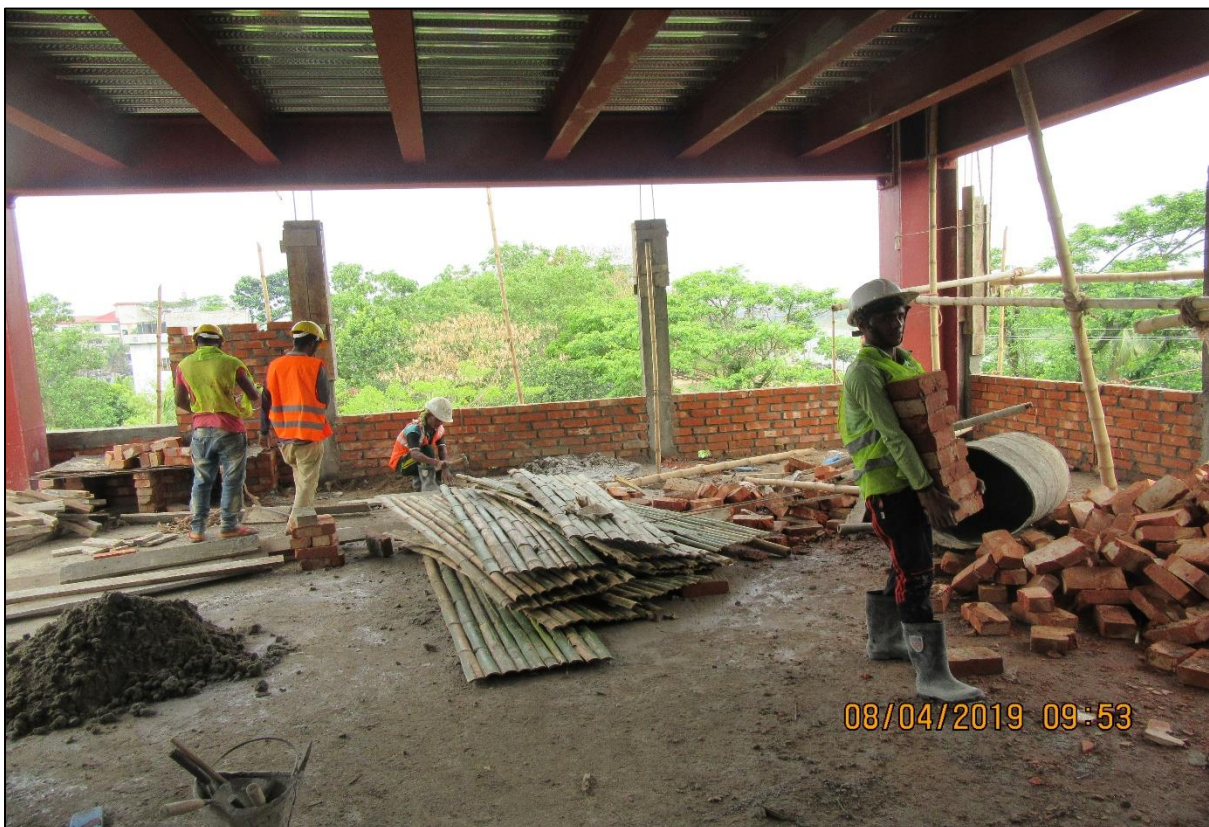
Figure 6: Construction of Command and Control Center and Warehouse of FSCD in South Surma, Sylhet.
