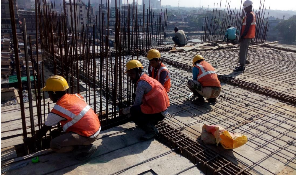
Figure 7: Construction of EOC in 5 th floor of Nagar Bhaban, Sylhet is ongoing
