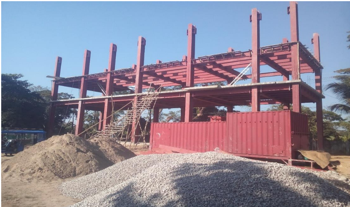
Figure 8: Construction of Command & Control Center and Warehouse of FSCD in South Surma, Sylhet is ongoing.
